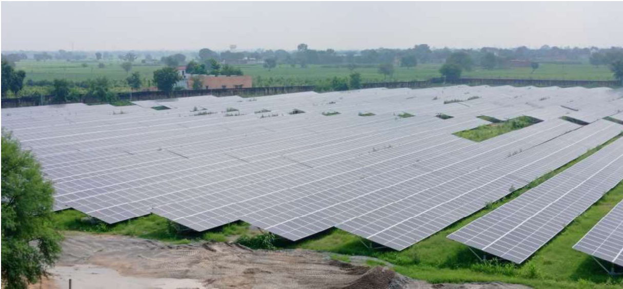
Solar Plant of 9 MW Commissioned in May -2022
